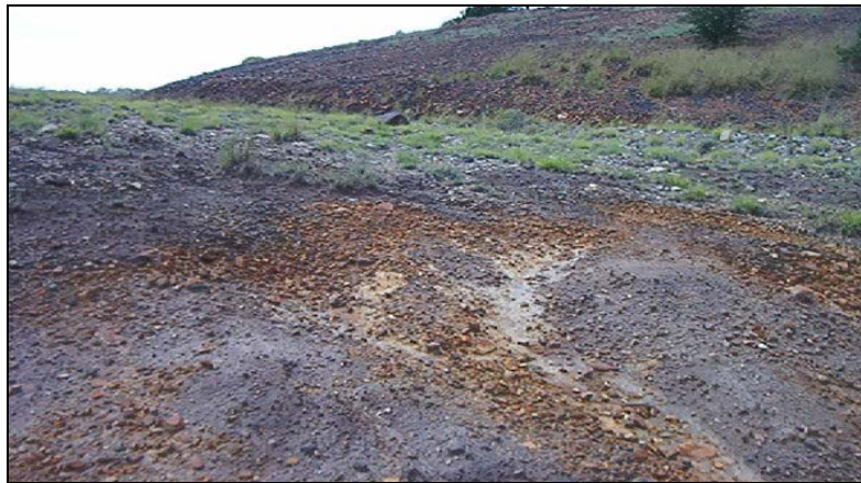
Photo 1. Obvious erosion on the east slope of Tailing Impoundment #3 (vegetation and soil cap have weathered away).
